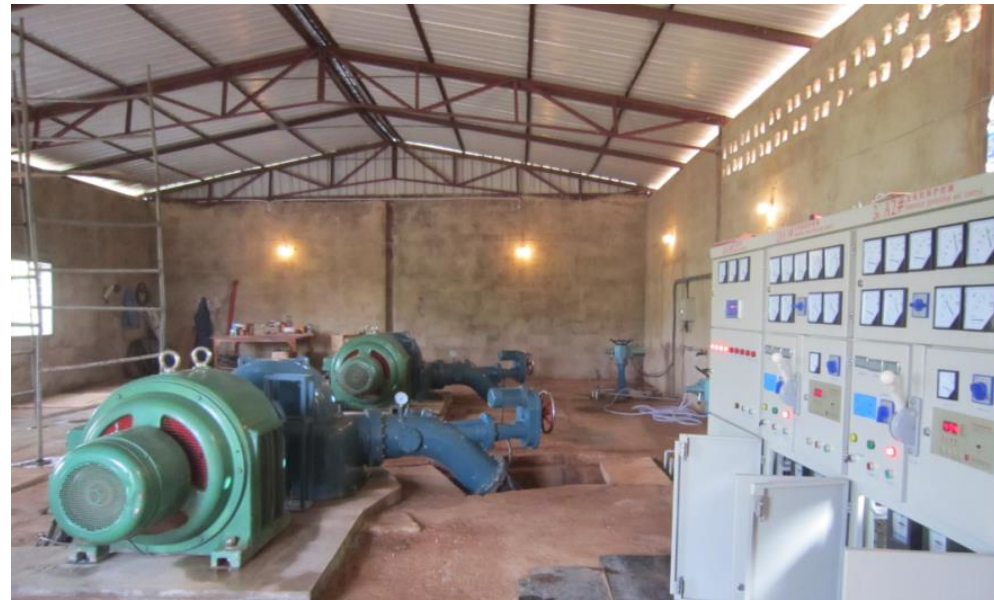
Two turbines of 200 kW each in Kakara, Highland Tea factory
